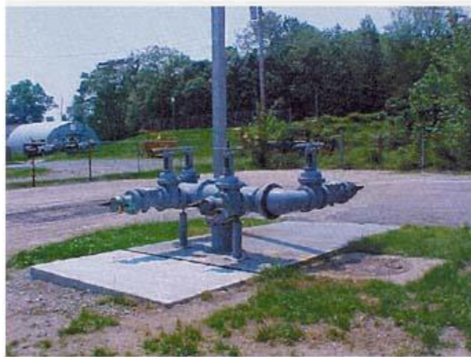
PS3 BYPASS PIPING TO CONNECT GODWIN PUMPS
