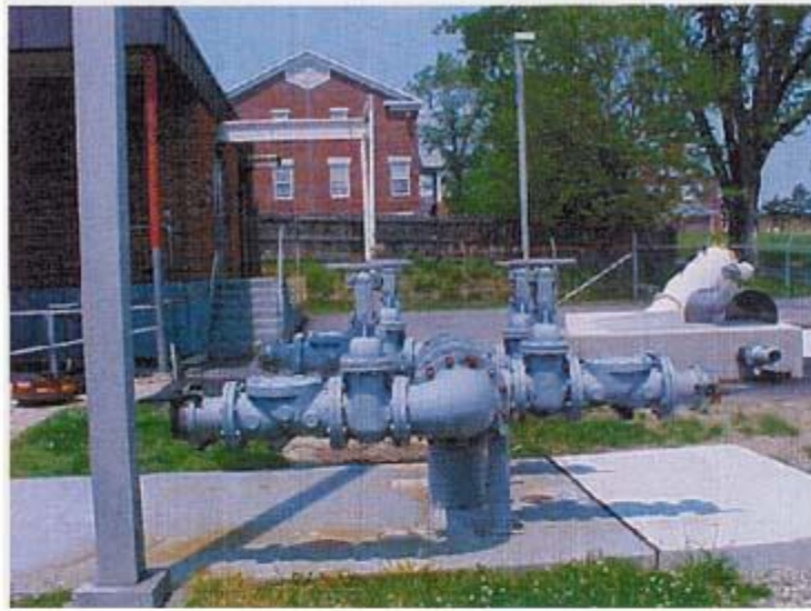
PS3 BYPASS PIPING
