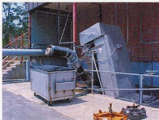
P83 FILTER SCREEN & DUMPSTER
