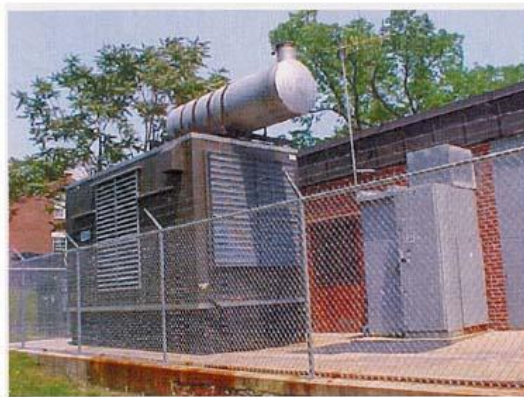
P33 EMERGENCY GENERATOR
